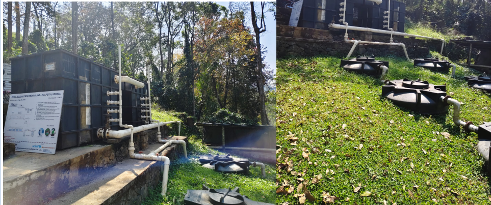
Faecal Sludge Treatment Plant
